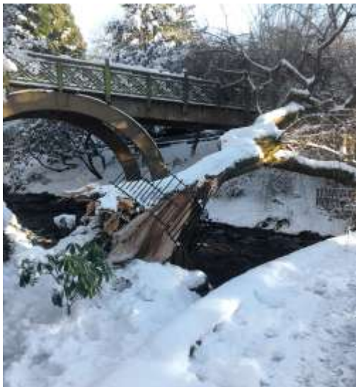
Storm damage at Crystal Springs.
